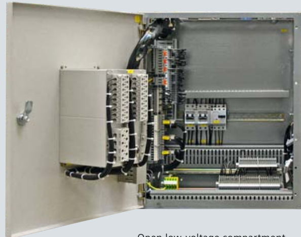
Open low-voltage compartment with built-in equipment (option)
